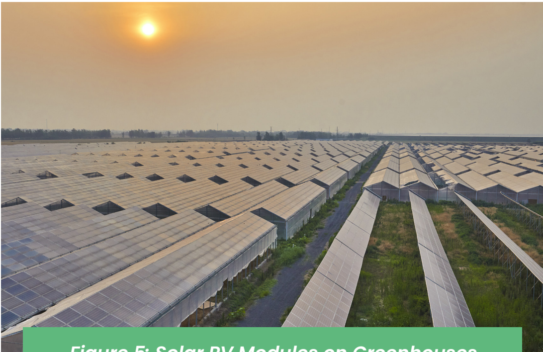
Figure 5: Solar PV Modules on Greenhouses
